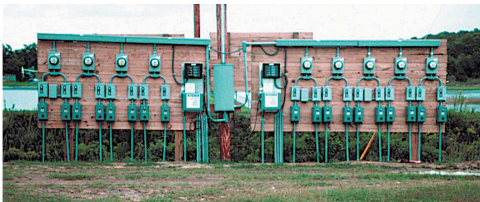
Control panels with automated system for controlling aerators based on dissolved oxygen levels.
