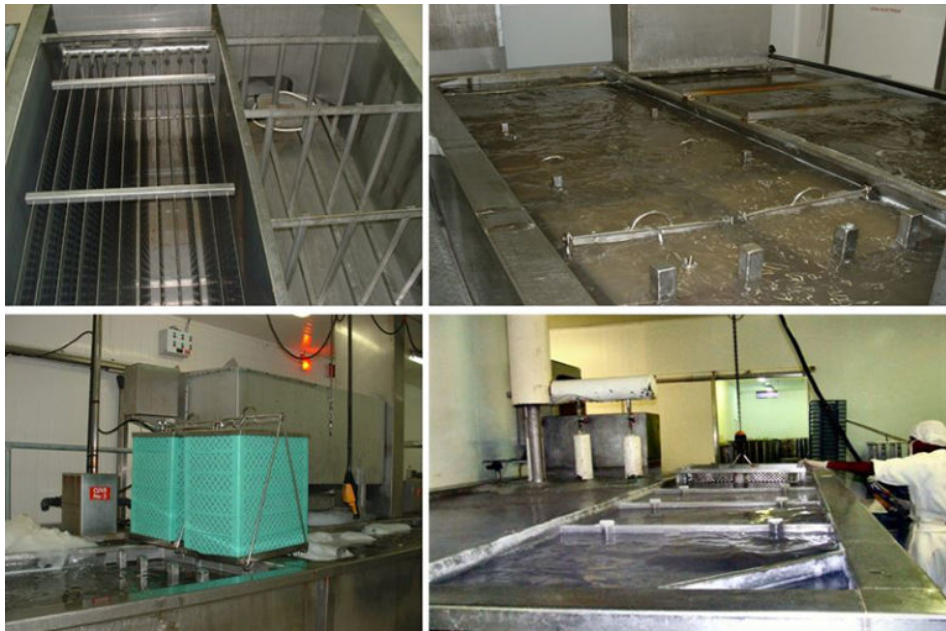
Views of empty and full brine freezers (top); dipping piles of shrimp blocks in brine freezing solution.
