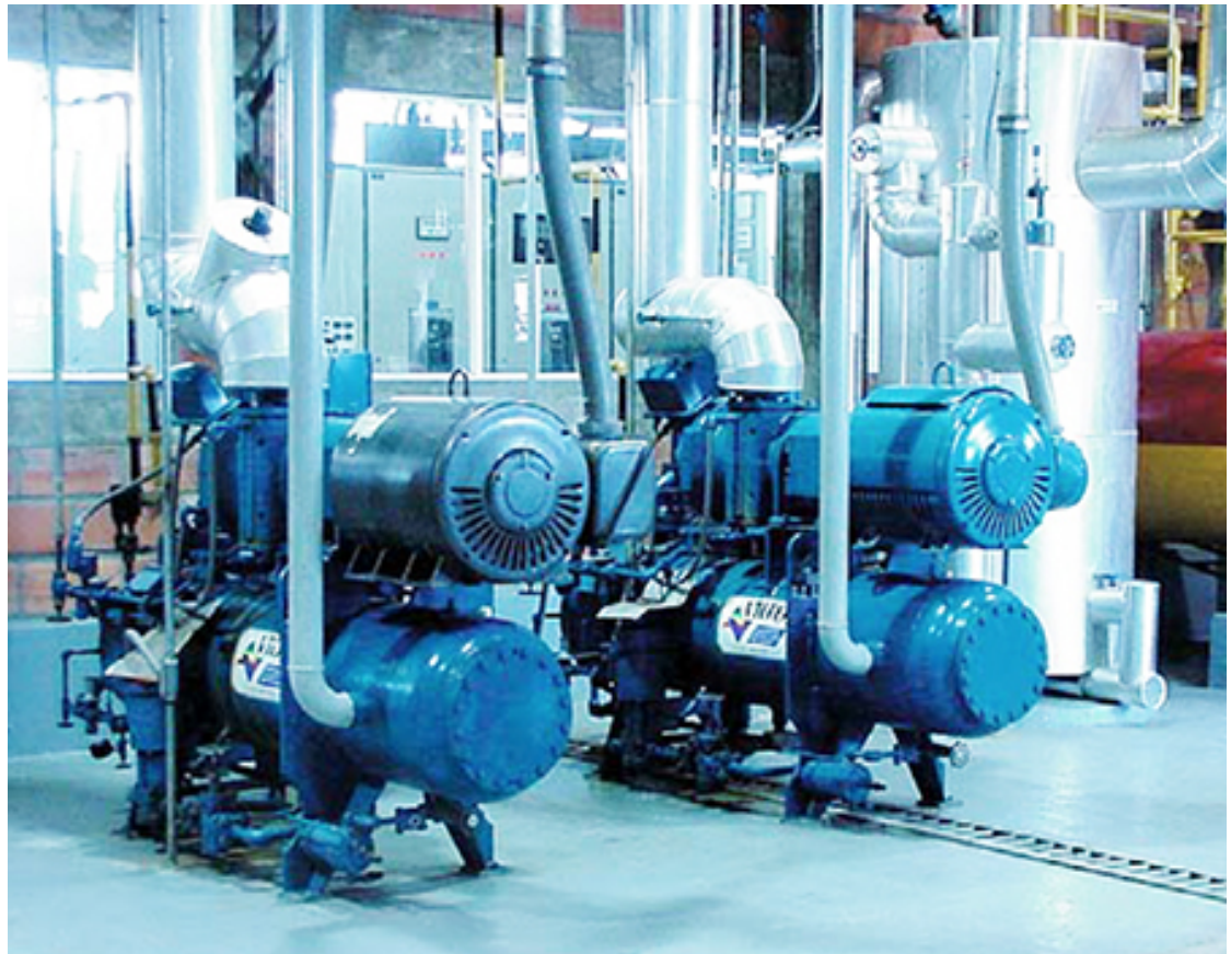
Ammonia-based refrigeration system. Photo courtesy of Vilter Manufacturing Corp.
