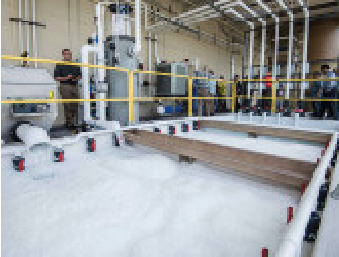
The biofilter media of this moving-bed reactor initially looks white and floats readily.
