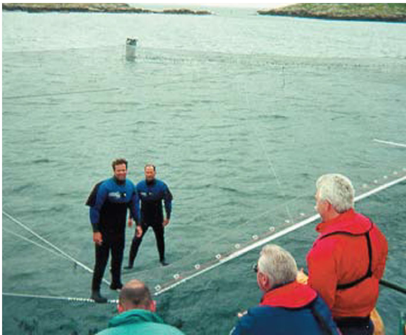
Fig. 1: A single 22,000-cubic-meter Ocean Spar in Killary Bay, Ireland. Installation engineers can be seen standing on the taut top net.
