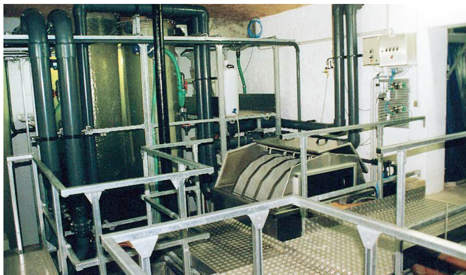
Recirculating water treatment system at an indoor fish farm in Germany.
