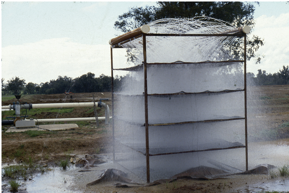
Well water that contains higher concentrations of ferrous iron can be treated by gravity aeration.
