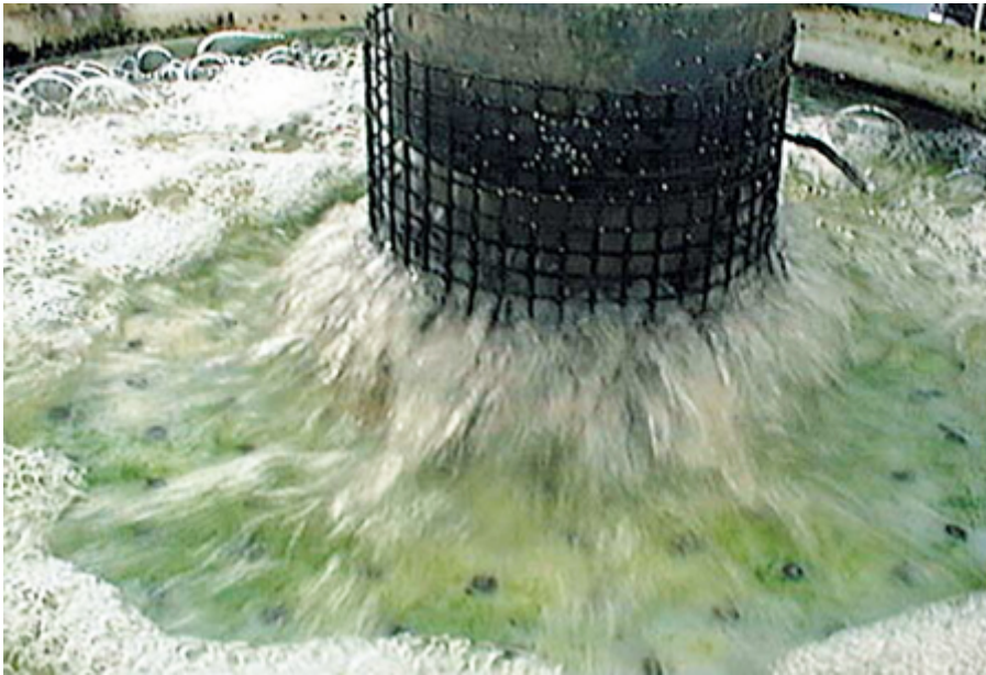
Packed column provides aeration at inflow into biofilter.
