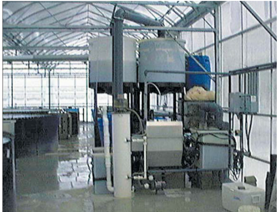
Biofilter complex at Target Marine in Sechtel, B.C. Canada.
