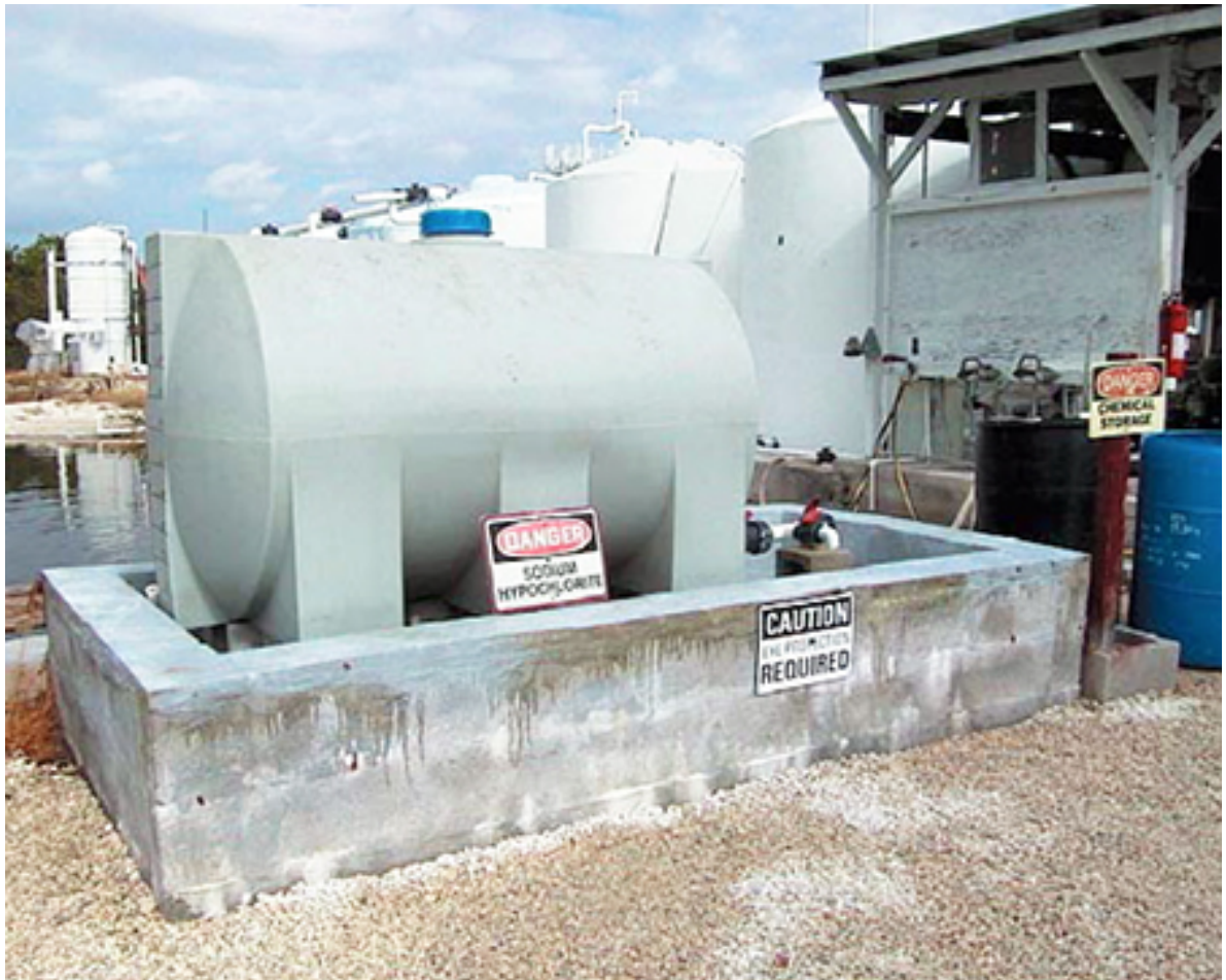
Secondary containment for chemical storage tanks minimizes the risk of accidental spills.
